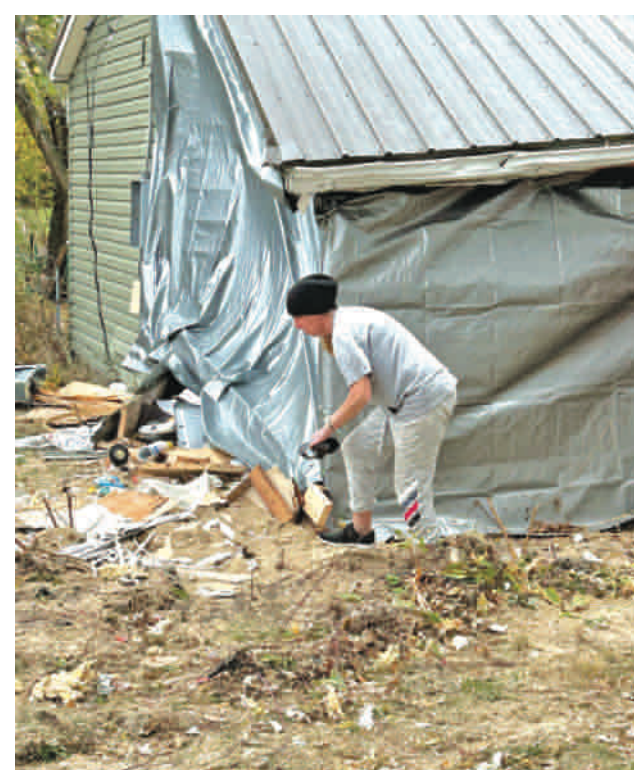
Tricia Hawkins begins picking up debris left behind after a semi crashed into her home. (EXAMINER PHOTO | TJ HUBBARD)
